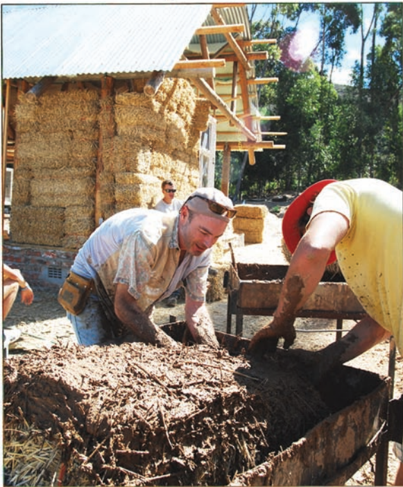
HANDS ON: Architect Andy Horn is not afraid to get his hands dirty when it comes to natural building processes.
